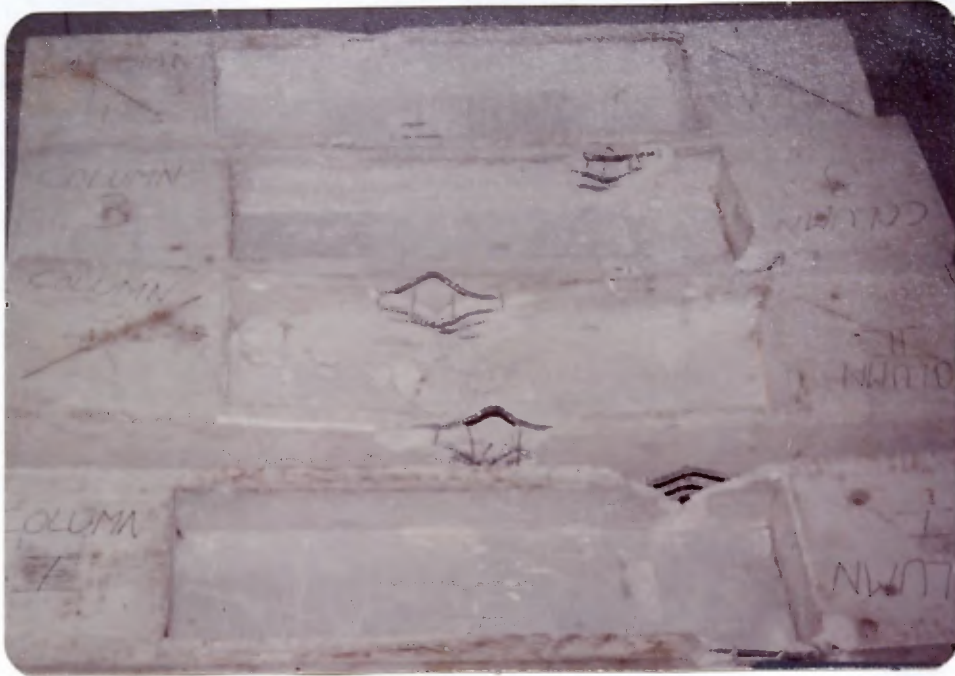
Fig. 3.4. Failure pattern in all Columns
